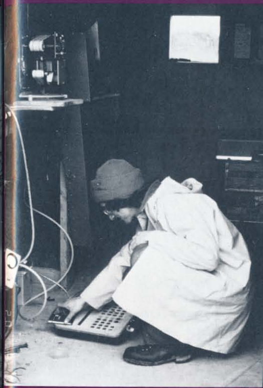
Telemetry system used for the stream and lake gages. Data from the gages are transmitted by satellite to Geological Survey offices in Vancouver and Tacoma, Washington. Technician Jonathan Brown is programming the GOES satellite transmitter which is coupled to the stream stage recorder. (Photograph by Terry Leighley, Sandia Labs.)
