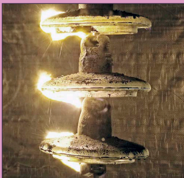
Flashover across a glass insulator string contaminated with 3 mm (0.1 in) of wet ash. Note the arc propagation over and through the conductive ash deposit. Photo by Johnny Wardman.
