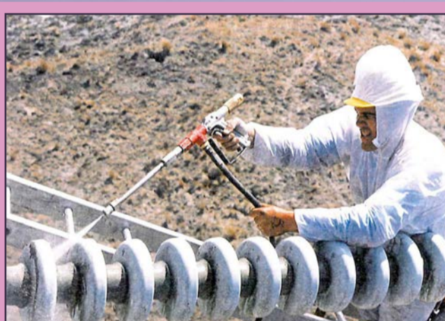
Ash from the 1995 eruption in New Zealand being cleaned from a 220 kV strain insulator. Photo by Transpower, New Zealand.
