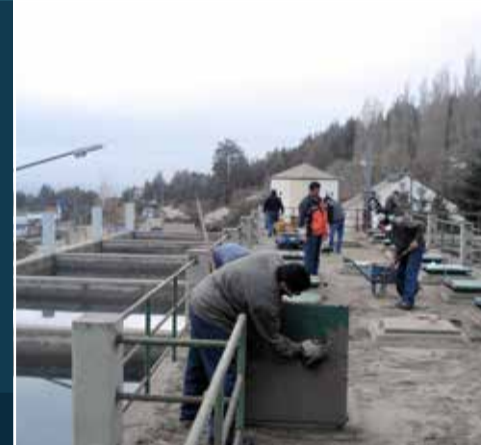
Ash can enter sand filter beds both from direct fallout, and through the intake. Cleaning of filter beds creates heavy additional labour demands, such as at Bariloche WTP following the June 2011 Puyehue Cordon-Caulle eruption (below)
